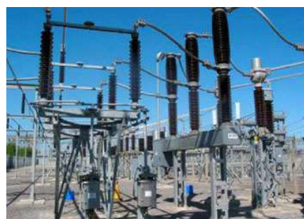
Basic and Detail engineering of electrical substations (up to 400 kV) RED ELECTRICA DE ESPAÑA
