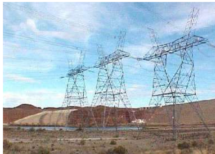
Basic and Detailed engineering for power supply to industrial facilities SEVERAL INDUSTRIAL CLIENTS
