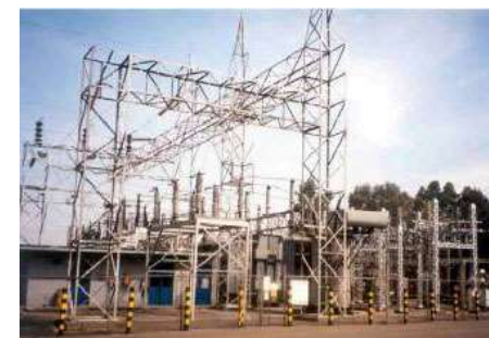
Detailed engineering of several Substations for Endesa: extensions, new transformers, new switchyards ENDESA
