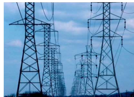
Basic and Detail engineering of high-voltage power lines RED ELECTRICA DE ESPAÑA
