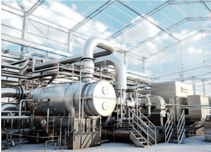
ISOLUX CORSAN 43 MW BIOMASS FIRED CHP PLANT Meta - Republic of Colombia
