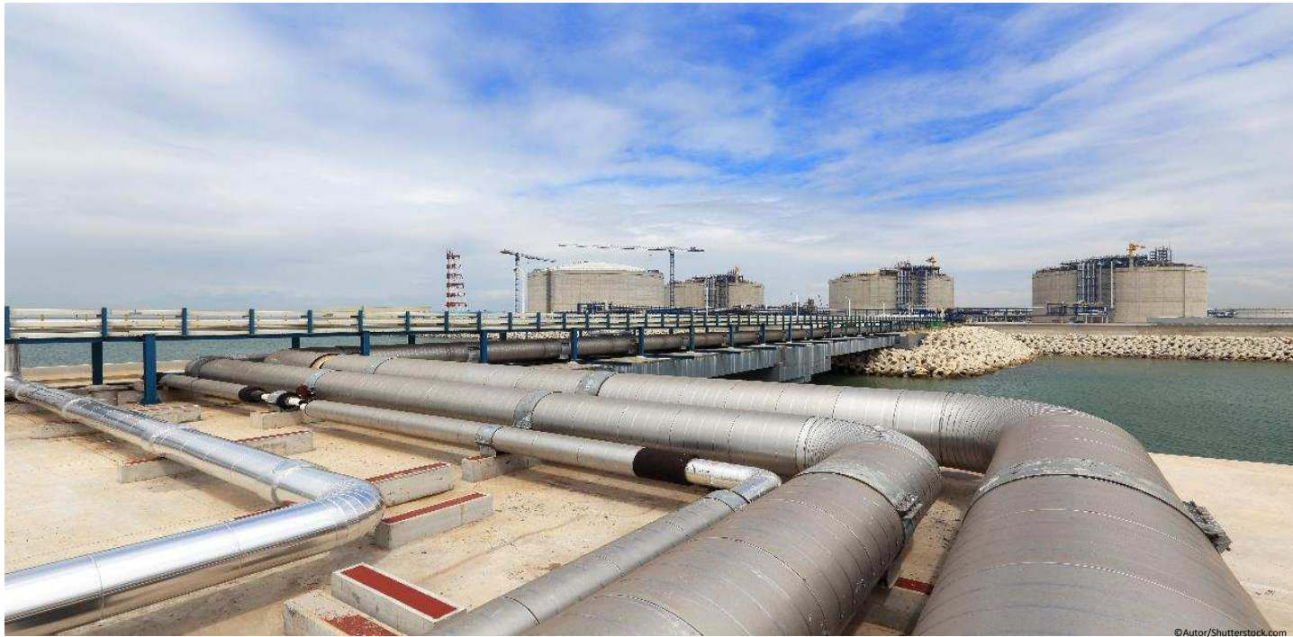
Gas treatment plant, LNG Terminal and liquefaction (Brazil)
