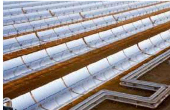
50 MW MORON CSP PLANT(SPAIN) Client/Owner ACCIONA_SERIDOM/IBEROLICA Parabolic trough technology with 96 loops EPC Power Block
