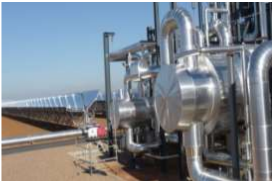
50 MW LA ARENALES CSP PLANT(SPAIN) Client OHL - MAN SOLAR MILLENIUM Parabolic trough technology Basic and detail design power block and HTF
