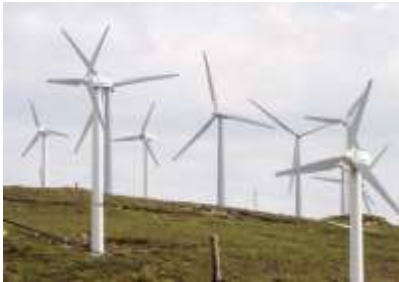
Wind farm 44 MW in Jerez Andalucia WIGEP ANDALUCIA
