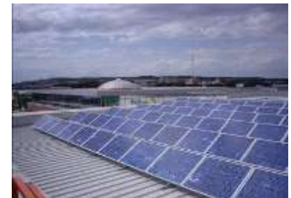
100 kW photovoltaic rooftop in Zaragoza Aragón TRANSPORTES OCHOA
