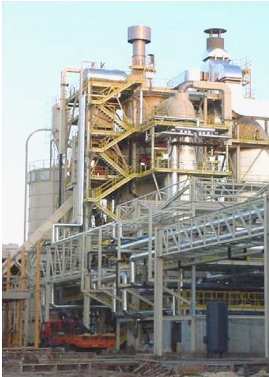
TAFISA 4 MW BIOMASS CHP PLANT Jaén - Spain
